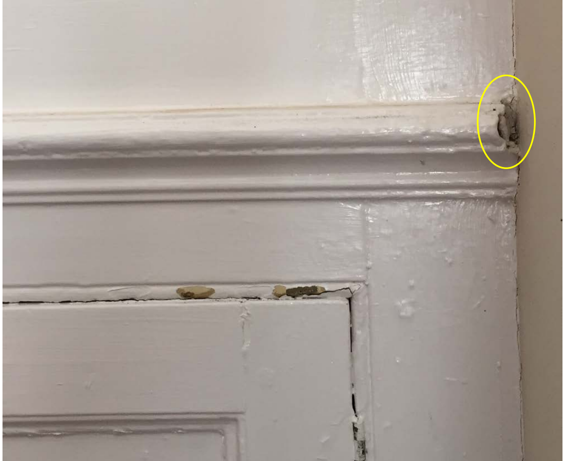
Figure 8. Detail of cabinet, showing former mitre joint between the chair rail on the cabinet and the non-extant chair rail that ran along the west wall (2016).
