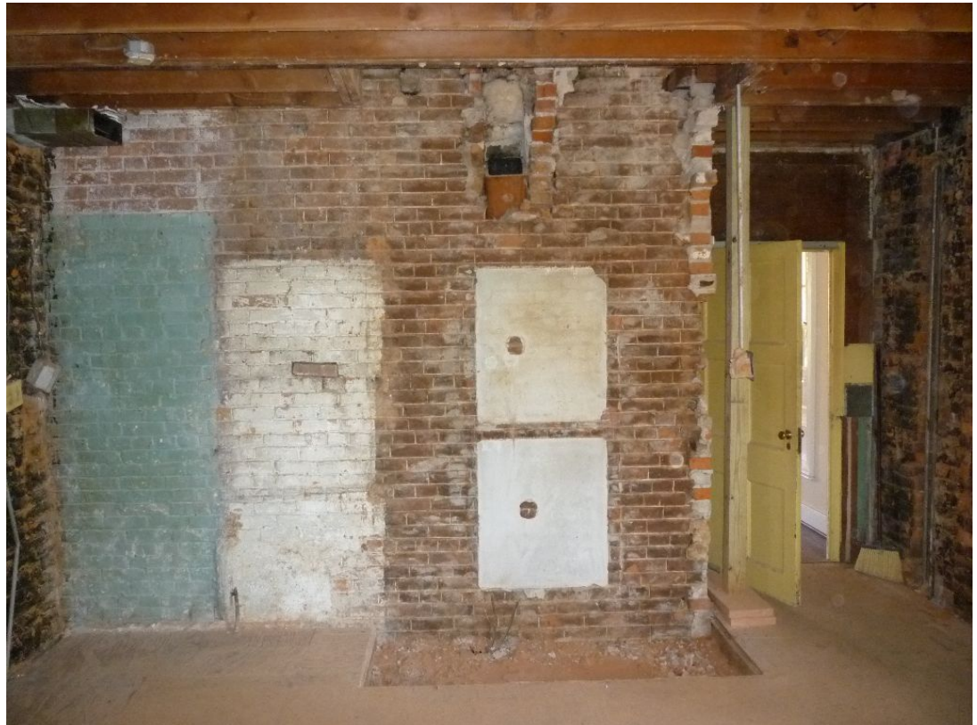
Figure 17. The former kitchen (Room 106) after demolition of the finishes. View looking north into Room 105 (2016).
