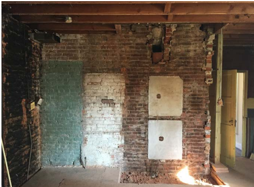
Figure 14. The north wall of Room 106, formerly the south exterior wall of the Period I Room 105; after removing 20 th -century metal lathe and plaster, and the brick base that had been installed to support the chimney when it was shifted slightly to the south when the room was converted into a kitchen in 1954 (2016).
