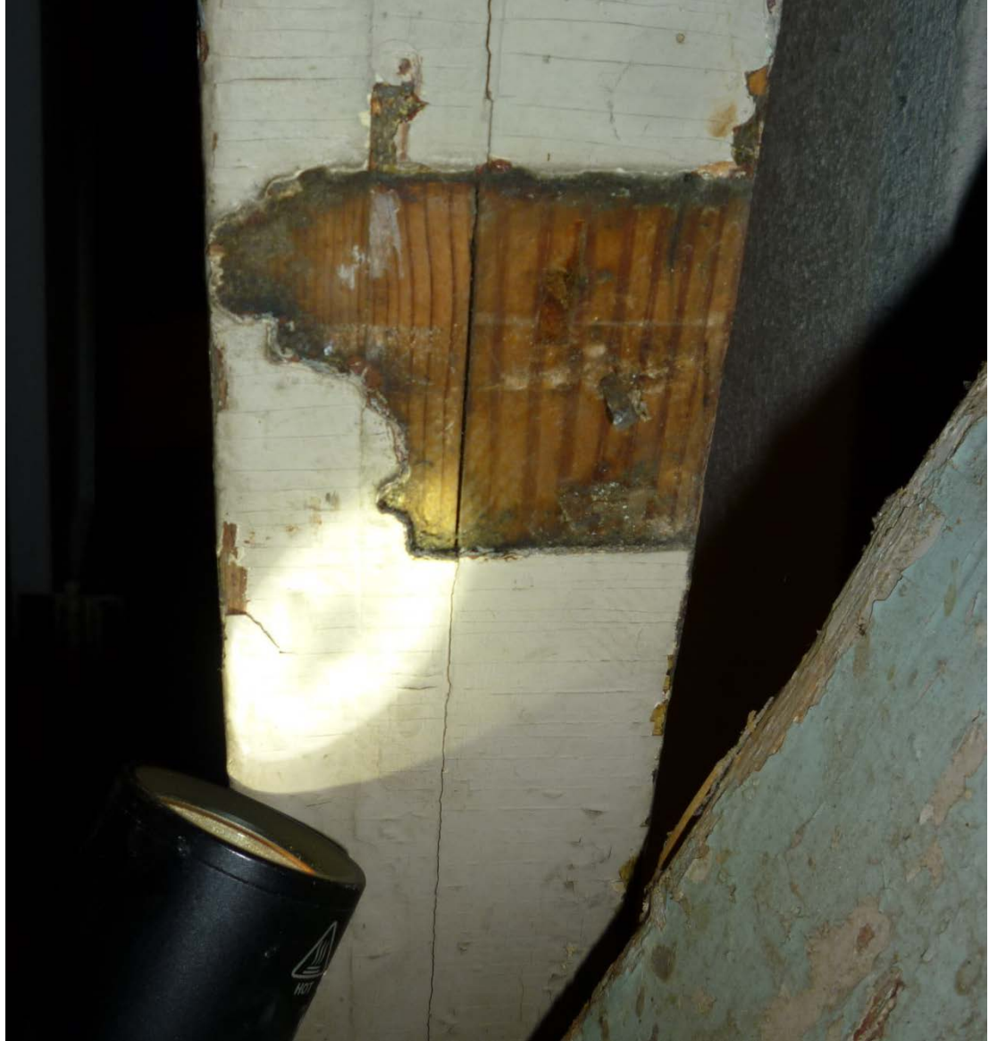
Figure 17. Paint ghost on detached mantel, which matches the profile of the chair rail found in Room 105 (2016).
