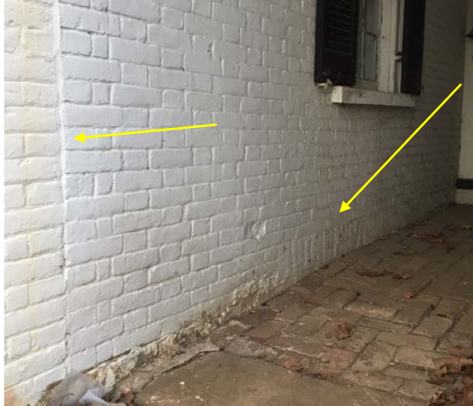
Figure 10. East wall of Period I section of west wing: vertical seam on left indicating junction of Period I and Period II construction; Flemish pattern brick bond; Period I window; soldier course of bricks below window at ground level, possibly indicating former location of bulkhead entry to the basement (2016).
