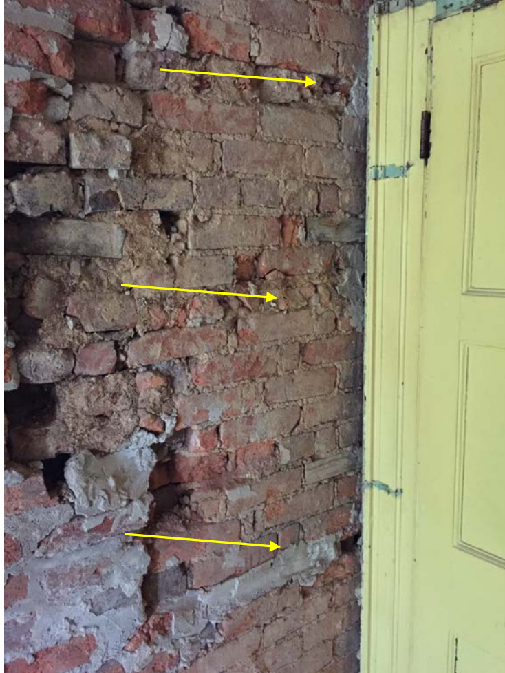
Figure 9. East face of Period I fireplace: on the left, scars from dismantling original south exterior wall; doorway inserted in Period II; three in-filled grooves cut into the masonry of the fireplace to support the ends of Period I shelves (2016).
