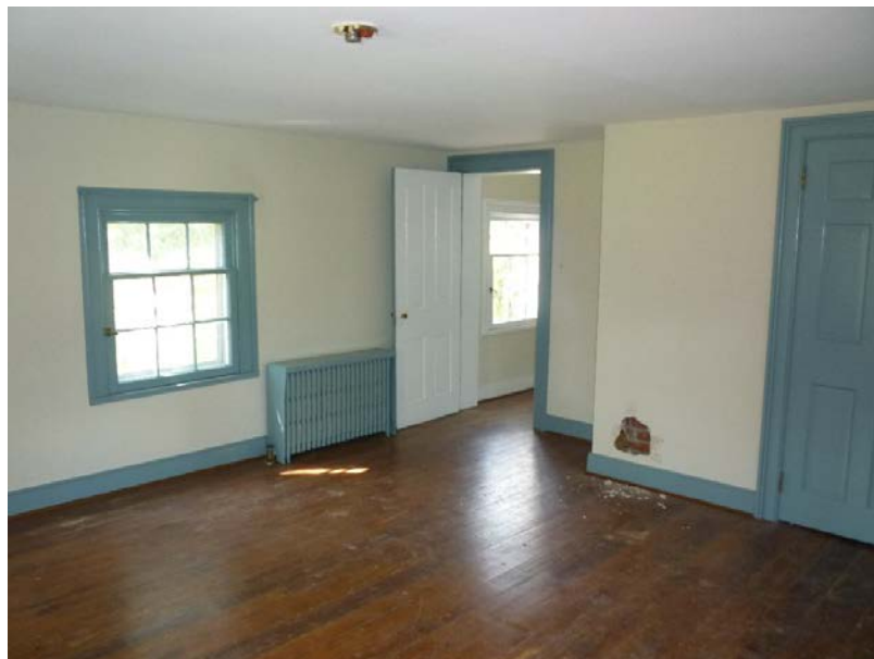
Figure 25. Room 206, looking northwest (2016). The brick flue next to the closet was removed by the FOHR in 2016.
